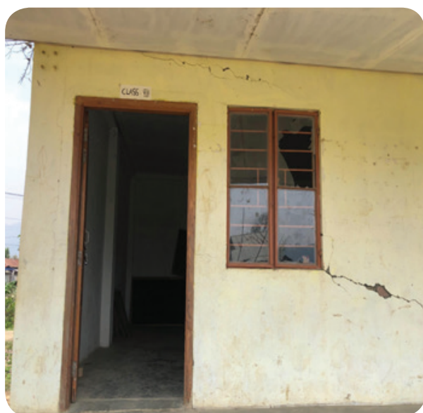
The dilapidated state of a classroom
